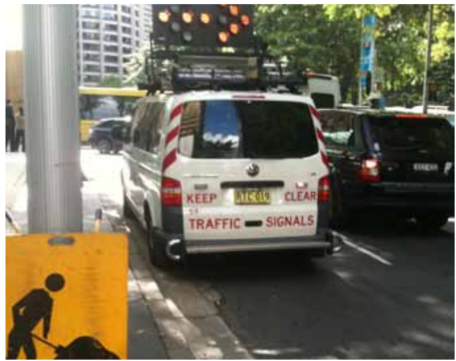
Figure 4: RTA cleaning traffic light lanterns at Wynyard Source: Mark Wolstenholme, NRMA Motoring & Services
