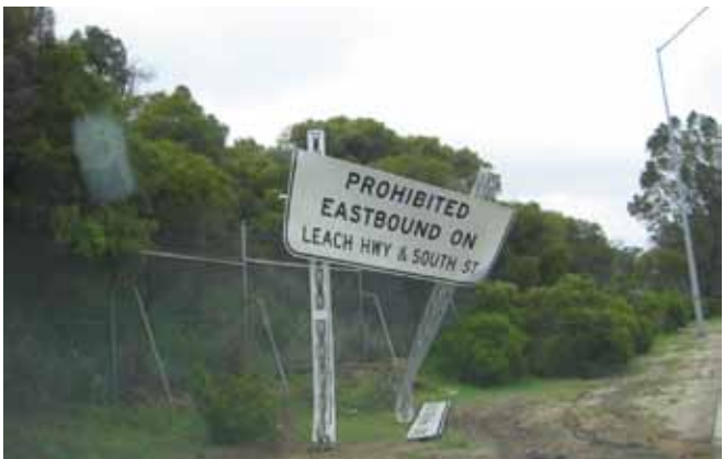
Figure 18: The first accident involving a UK-type sign post in Australia occurred when a vehicle travelling on the Kwinana Freeway south of Perth, Western Australia. No injuries were sustained in this crash. Photo courtesy of ASP Group Pty Ltd
